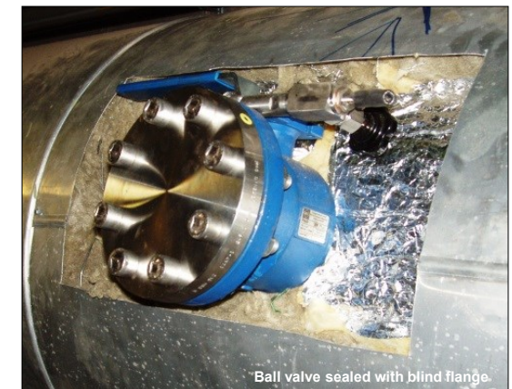
Ball valve sealed with blind flange.
